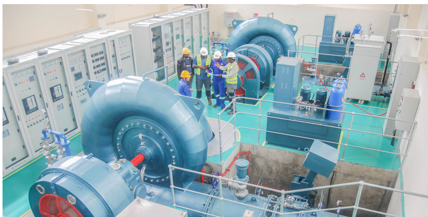
Kasanjiku mini hydro power station in Mwinilunga district, North-Western province
