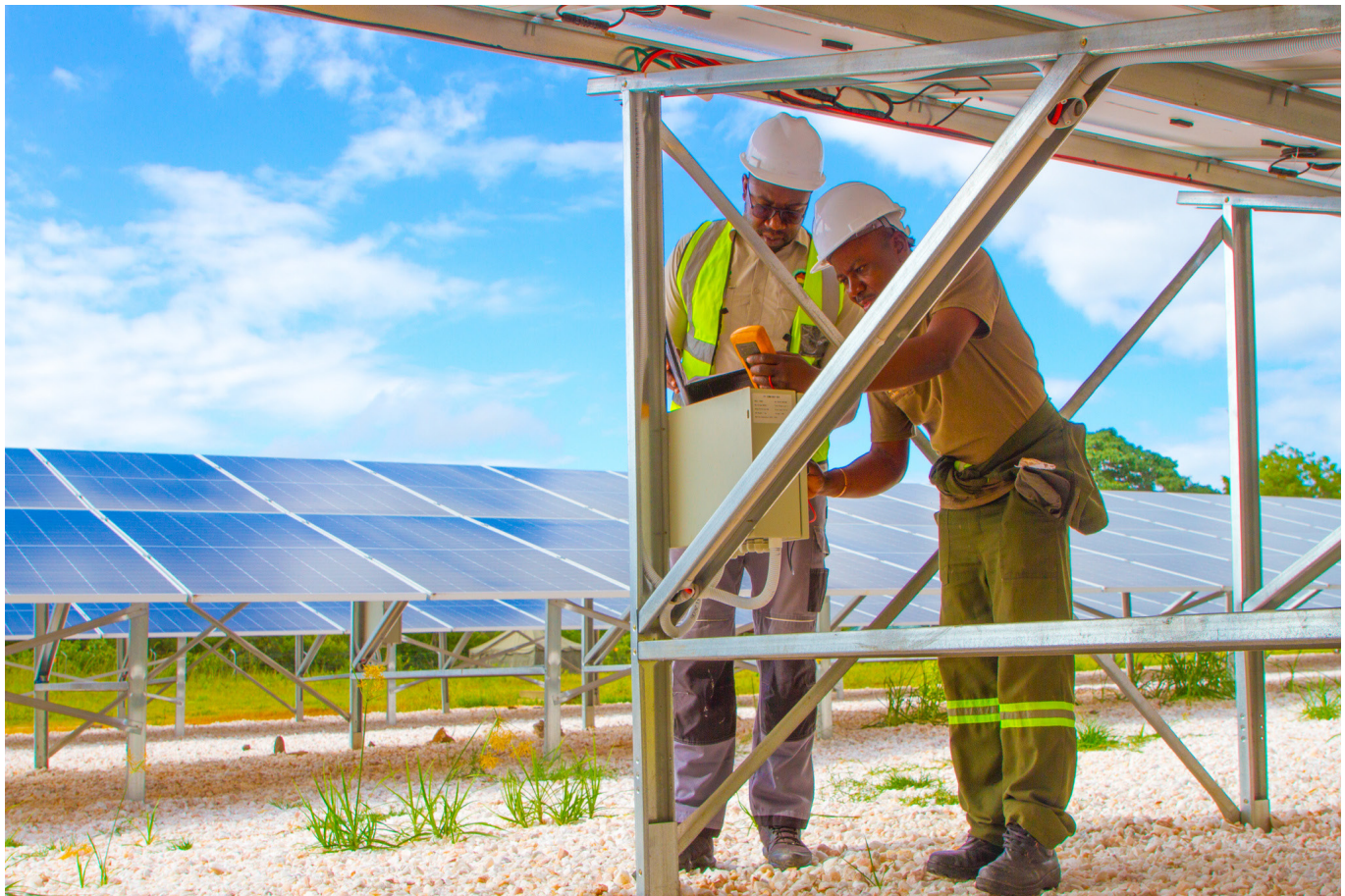
Solar panels at the Chunga solar mini grid project in the Kafue national park in Mumbwa district, Central province
