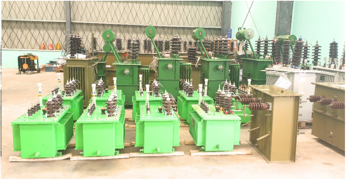
Transformers ready for delivery to labour-based project sites
