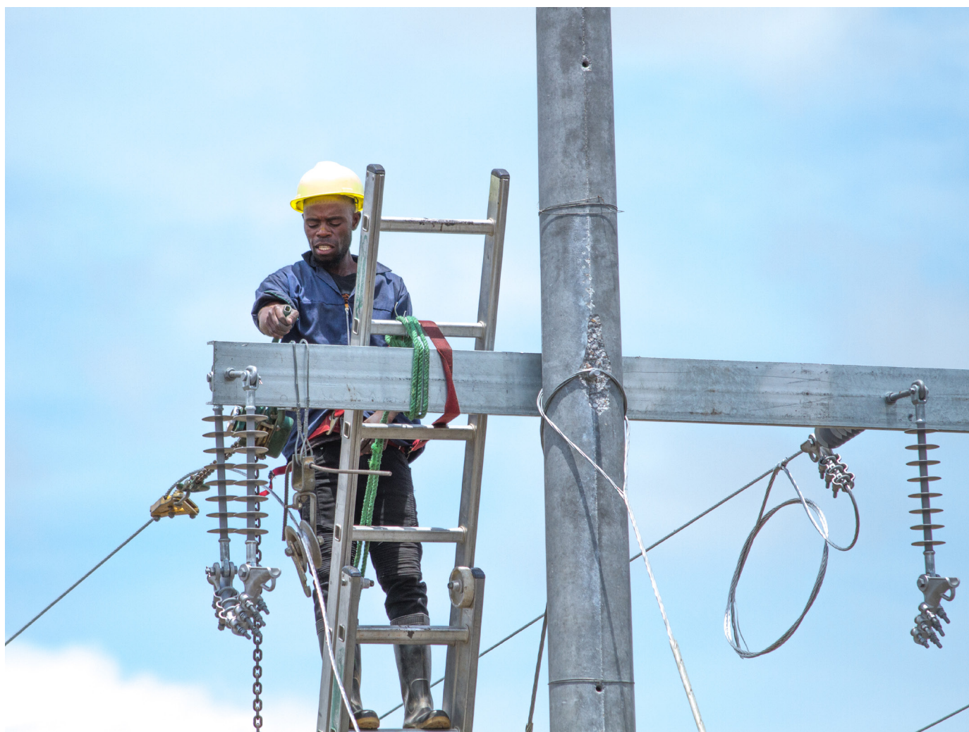
Construction of high voltage lines on the Chiefs in Itzhi- tezhi grid extension project in Southern province
