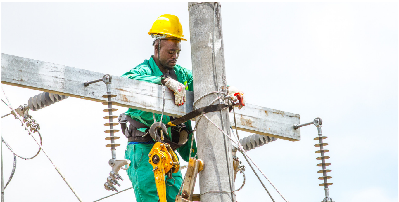
Construction of high voltage lines on the Chiefs in Itezhi-tezhi grid extension project in Southern province
