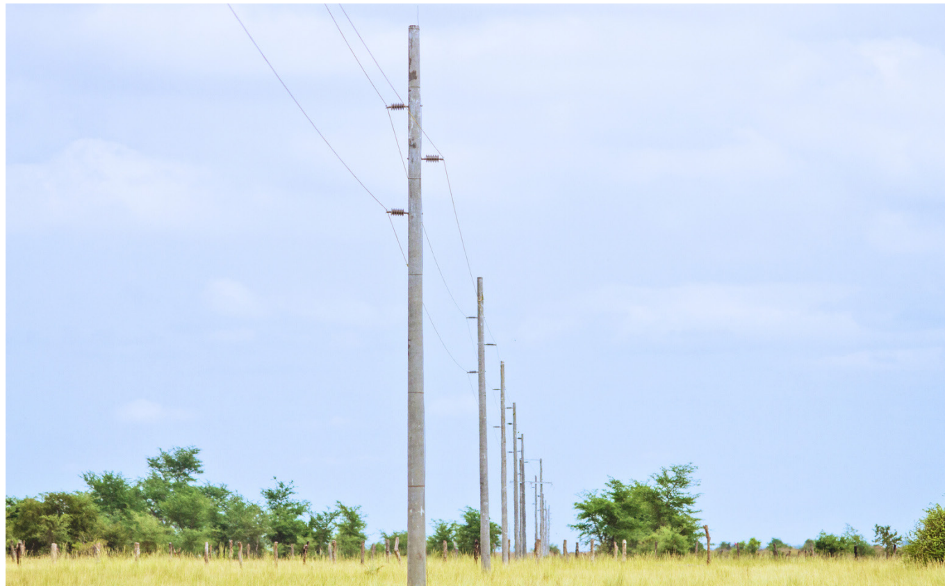
Part of the High Voltage lines on the Chiefs in Itezhi-tezhi Grid Extension Project in Itezhi-tezhi district in Southern province
